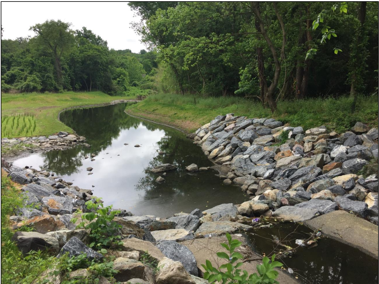
Recently completed stream restoration project. Rocks were used to stabilize the banks and fresh vegetation was planted along both banks.
