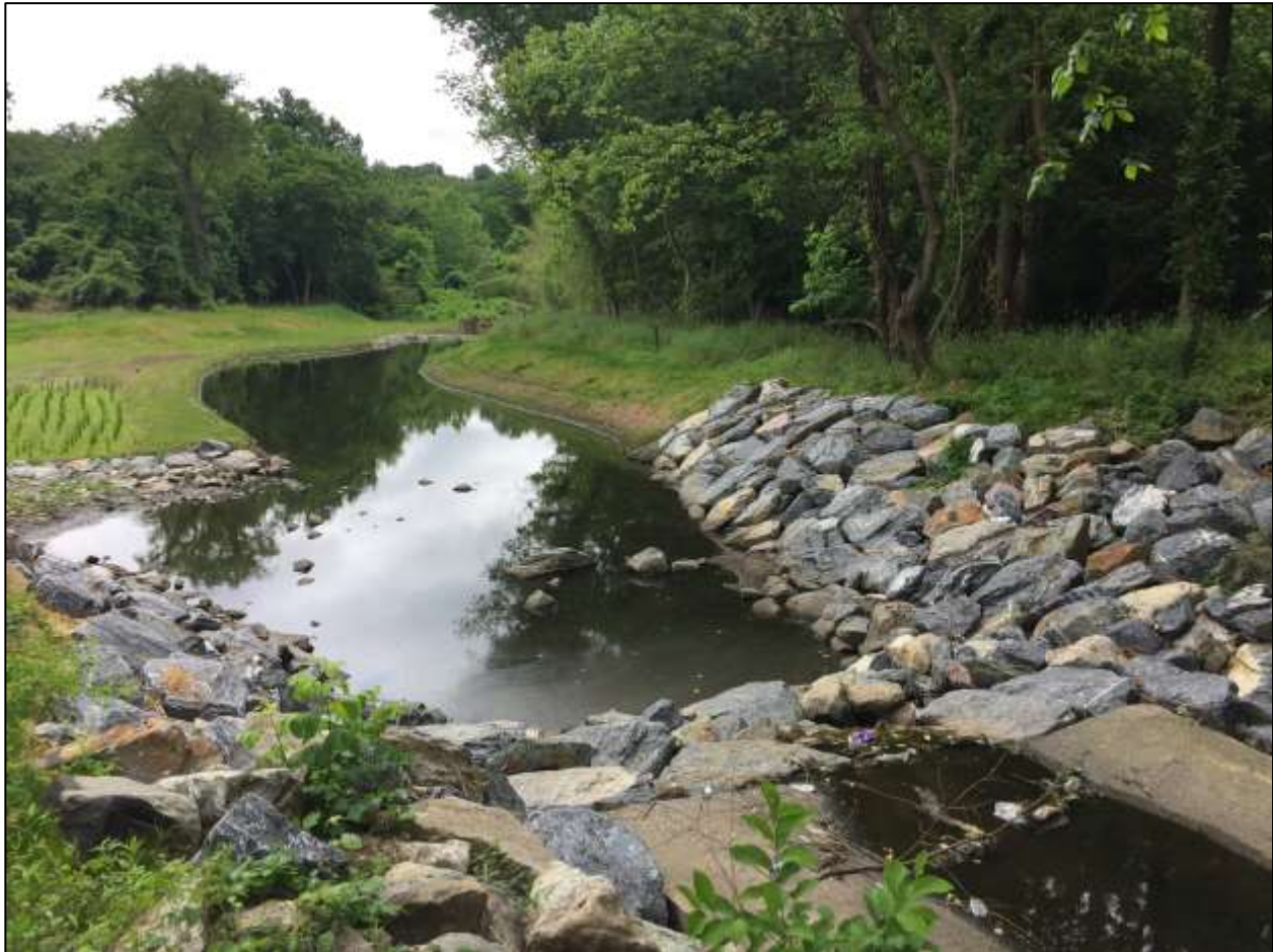
Recently completed stream restoration project. Rocks were used to stabilize the banks and fresh vegetation was planted along the left and right banks.
