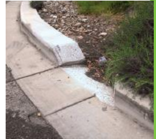
Curb cuts shunt runoff from roads and parking lots to pervious areas.
